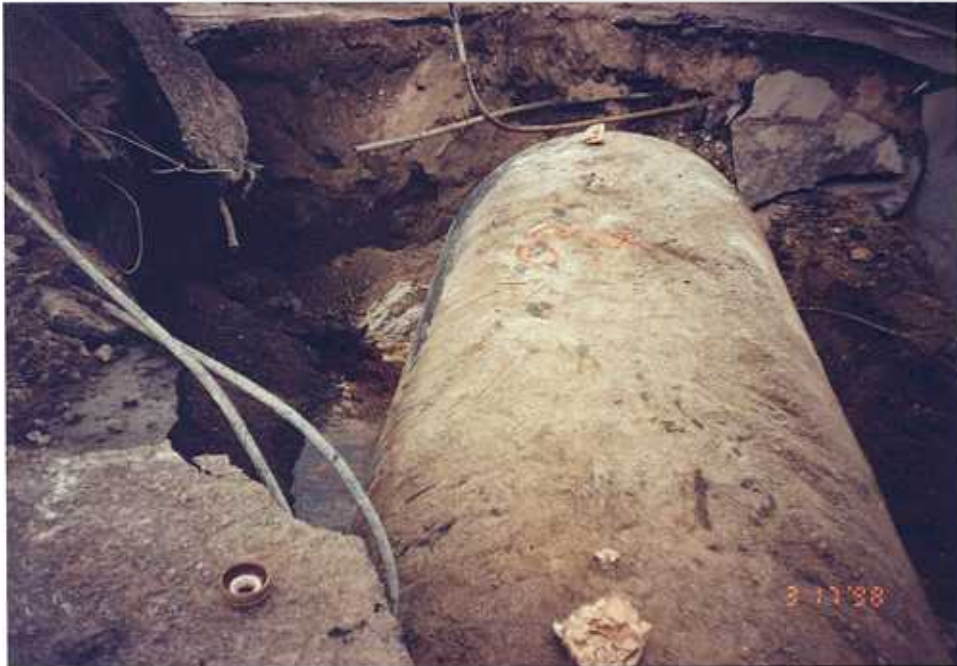
Above: Hydrocarbon sludge floating on groundwater left of the failed underground storage tank.
